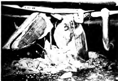
Photo 31. Shear failure of reinforced concrete column in ground story.
